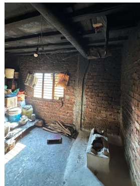
Soot-darkened kitchen interior
