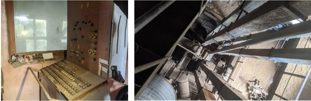
Picture 16 and 17: Palmse grain factory control panel and a dangerous state example
