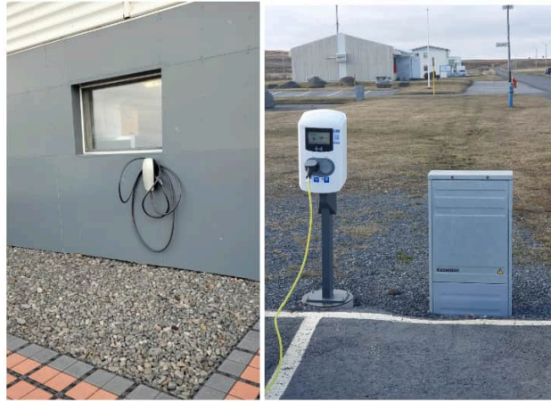
Fig.11. Electric car charging points
