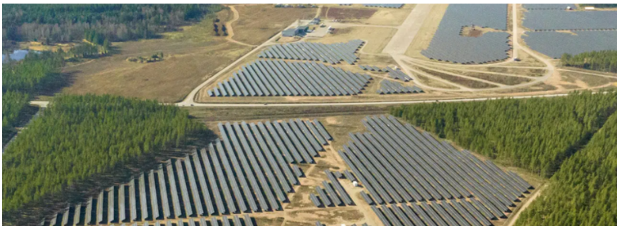
Figure 4. Sweden's Largest Solar Park. Hultsfred (Neoen, 2025).
